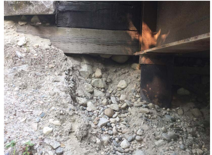
Erosion under ballast wall, both banks
